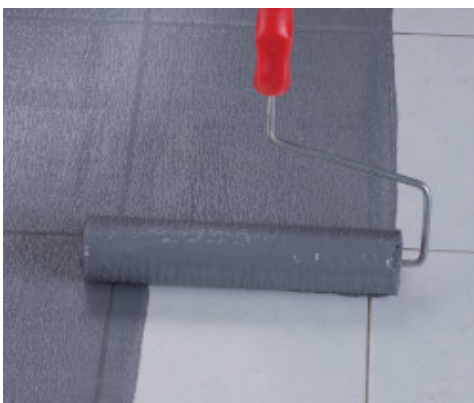
Application of Eco Prim Grip Plus by roller on existing porcelain tiles
